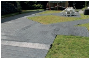
Figure 3: Wrong! Laying without expansion joints, tiles warp when exposed to sunlight
